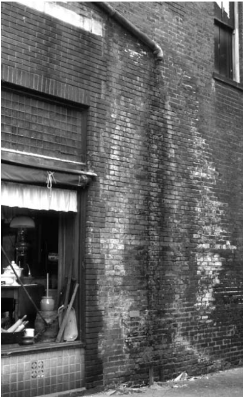
Both chemical salts (efflorescence), which leaves white residue, and mold or moss can grow on old buildings when a broken downspout allows water to shed over a portion of the building's exterior. Damage to interior plaster and wall finishes also can result.
