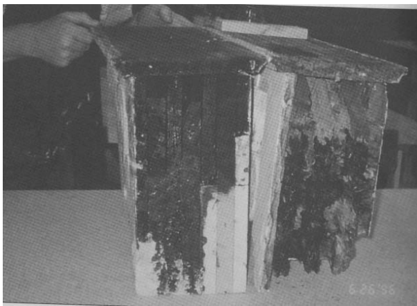
Before and after views of a deteriorated bracket. The bracket on the left was repaired through the use of consolidating epoxy as well as dutchmen.
