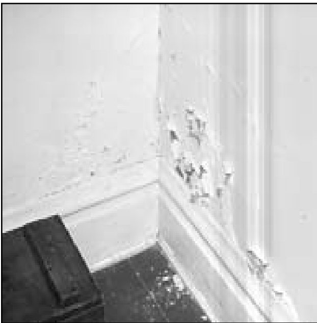
Typical plaster damage that can occur inside a building.
